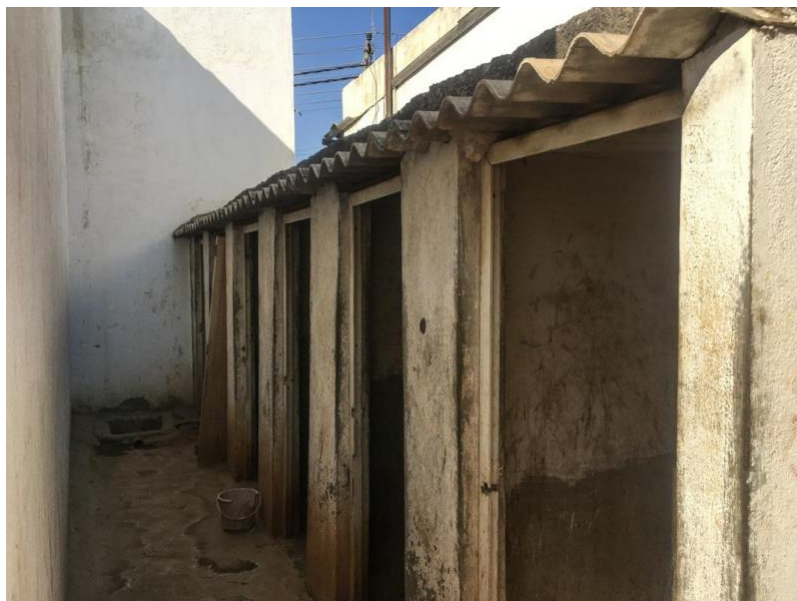
Bathrooms do not have doors. Of the four bathrooms, only two are functional. The rest are clogged and have not been cleaned in months. This has to be shared between 200 workers.
