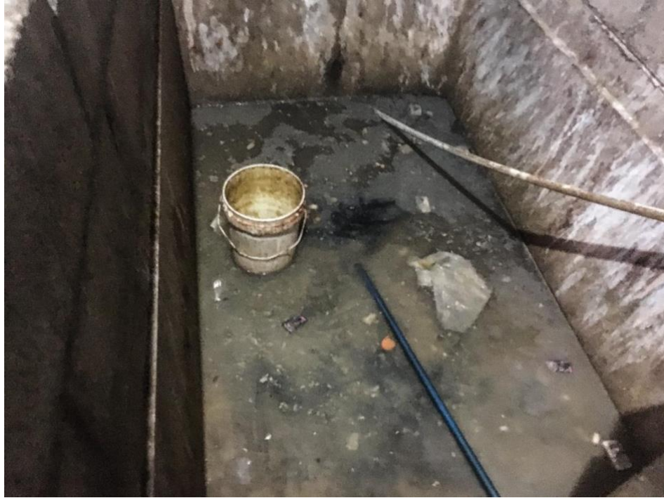
The bathroom is clogged for several days now. It is practically unusable. There are only two bathrooms in this colony.
